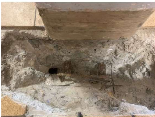
Sondage SP-4 – Surface plancher
